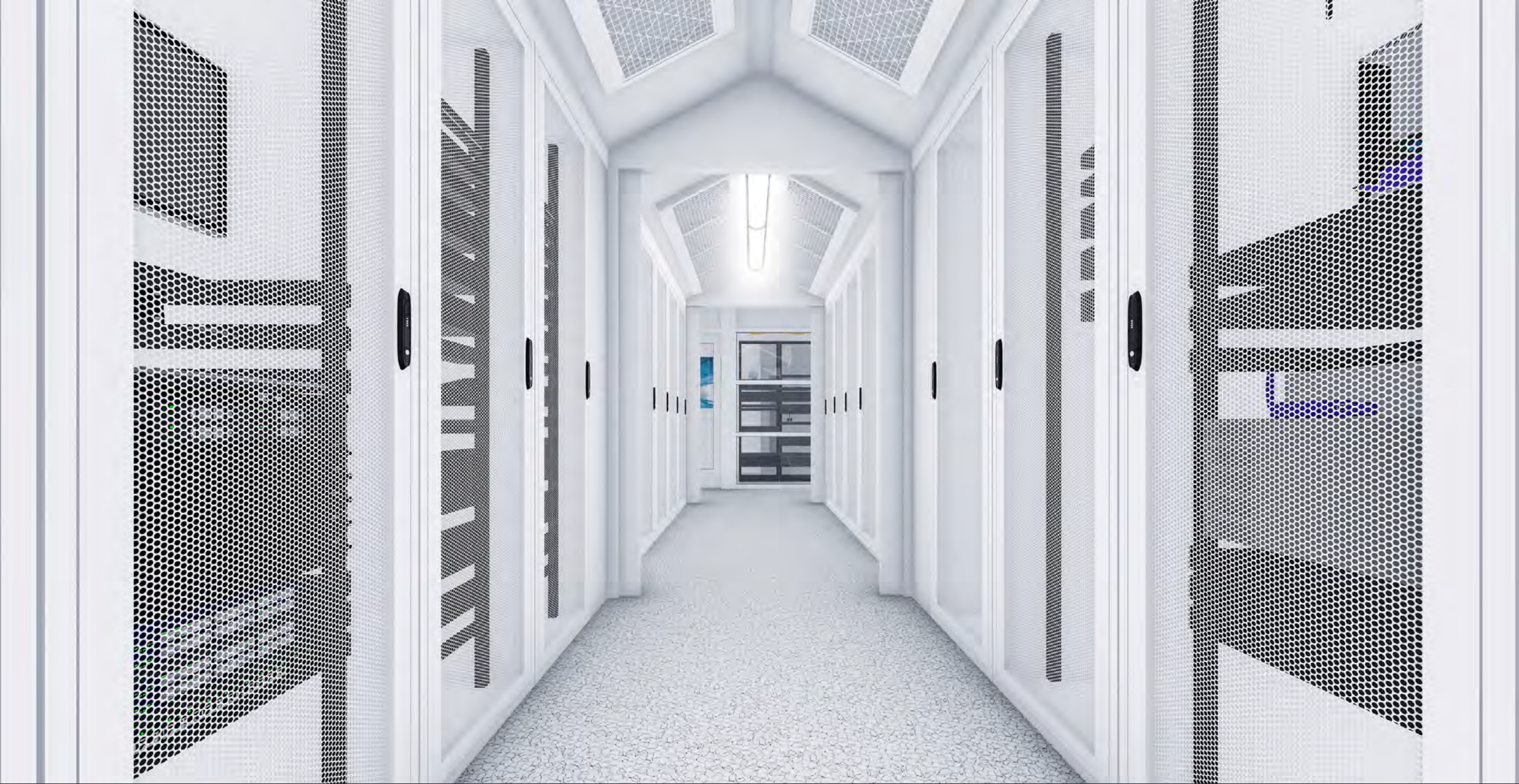
Colocation Cabinets (hot aisle side, with chillers above)
